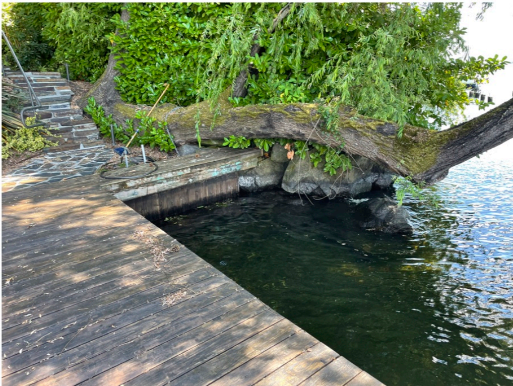
Photo 4 - Shoreline conditions looking south of the dock. Bulkhead to be replaced.
